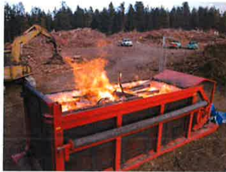
Figure 1—ACD in full operation (no visible smoke).
