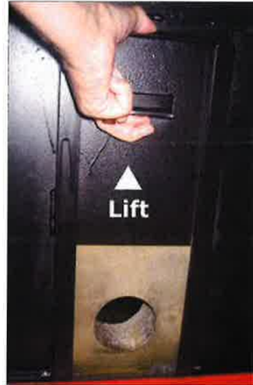
Access Door for Lighting
